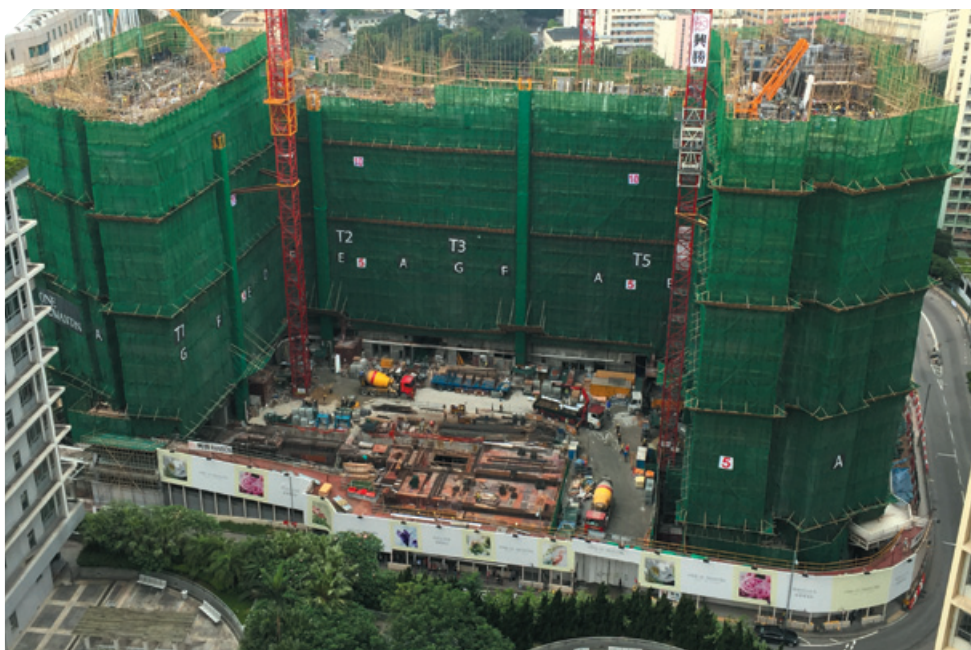
Proposed residential development at 1 Sheung Foo Street, Homantin, Kowloon 九龍何文田常富街1號建議住宅發展項目
